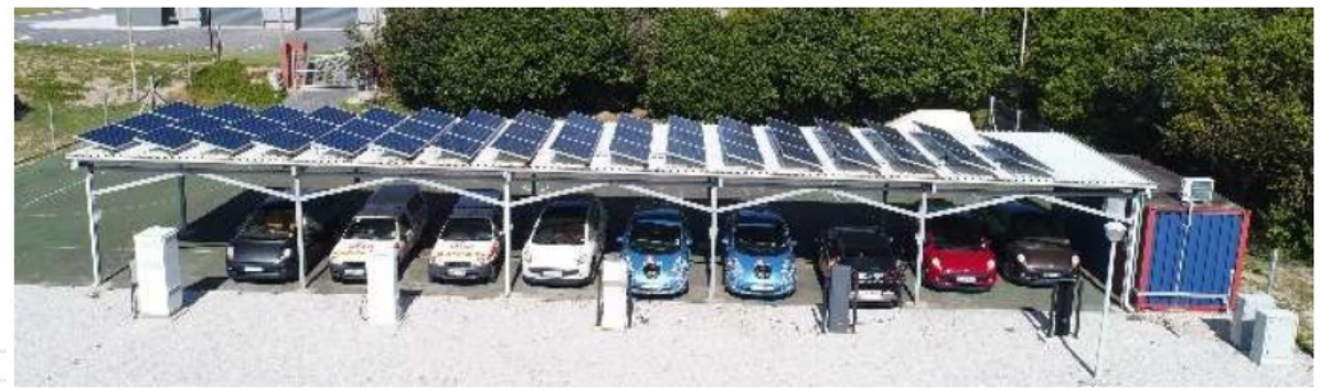
uYilo Smart Grid area based at North campus
